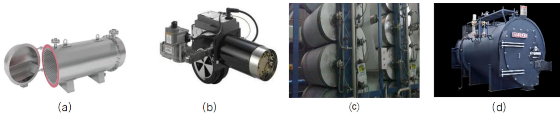
Fig. 9. Facilities of dyeing and finishing process using steam and LNG; (a) heating apparatus for a dyeing machine (shell-and-tube heat exchange), (b) tenter machine, burner for dryers (lng burner), (c) can dryer (using steam), (d) steam boiler. KTTA (2023), p.16~27.
